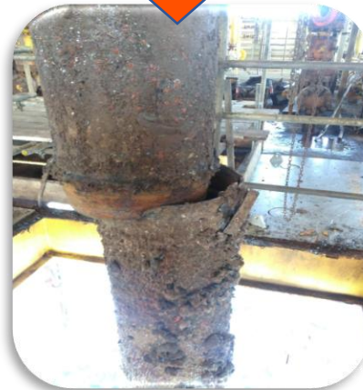
20" conductor installed in late 1980's
