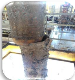
Failed 20” conductor couplings
