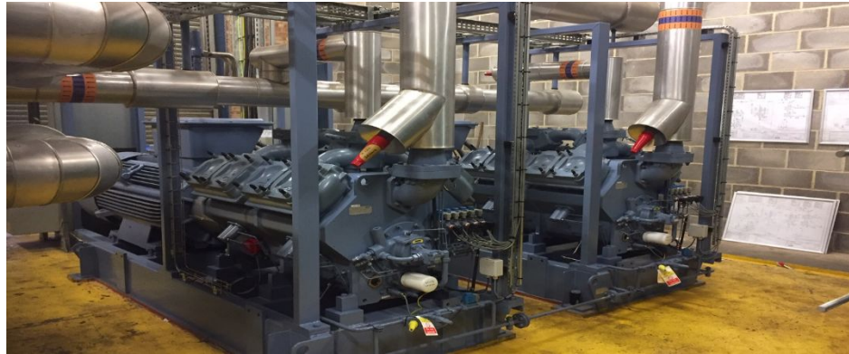
Heat pumps at Abbotsford Road. Photo by © Jonathan Steven
