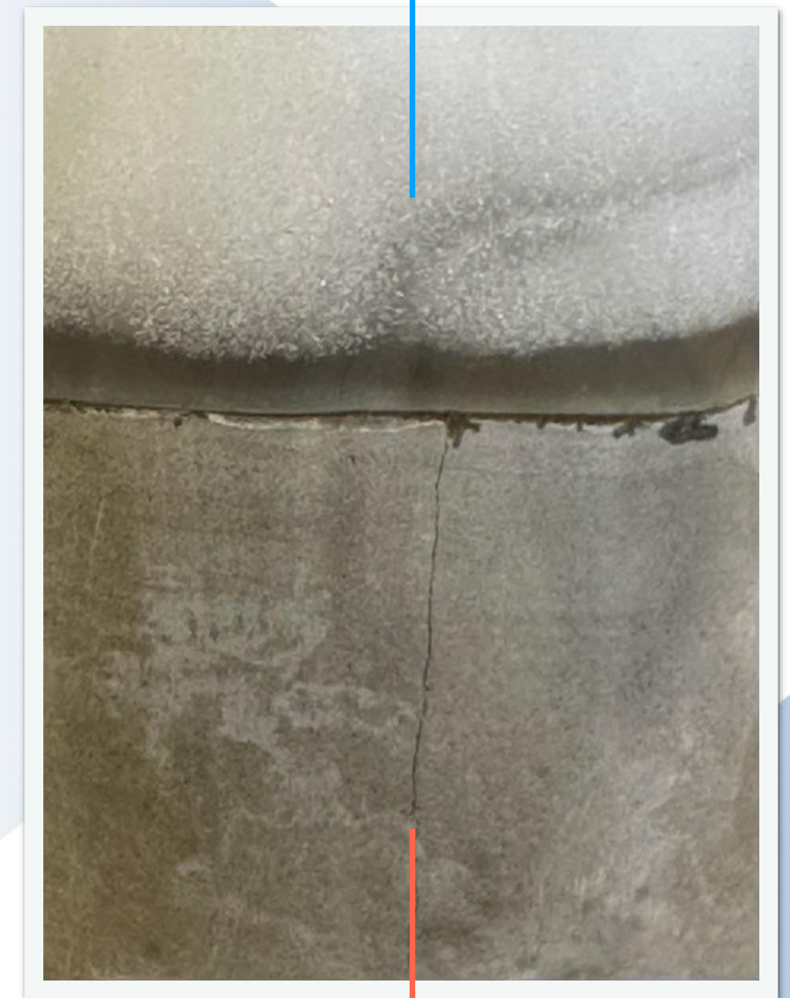
Solid State Barrier - crack formed in cement
