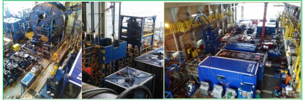
Multiple equipment packages on deck for B09
