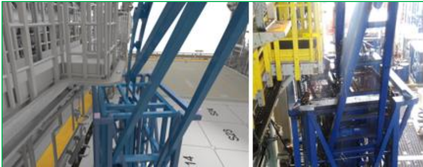
Use of 3D model to identify clash of CT injector and jacking frame
