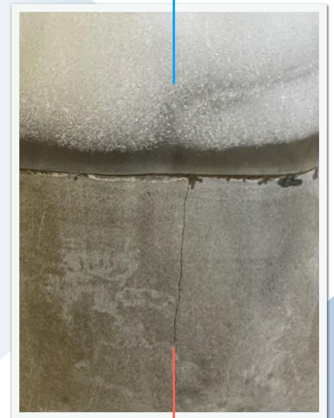
Solid State Barrier - crack formed in cement
