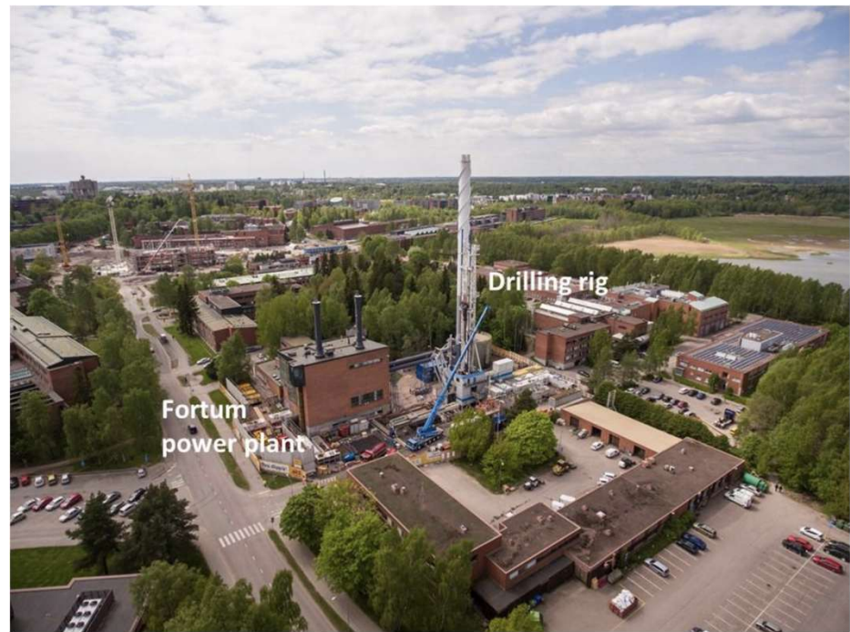
Set up of drilling rig on site in Espoo, Finland. (EGS research project) (Source: St1)
