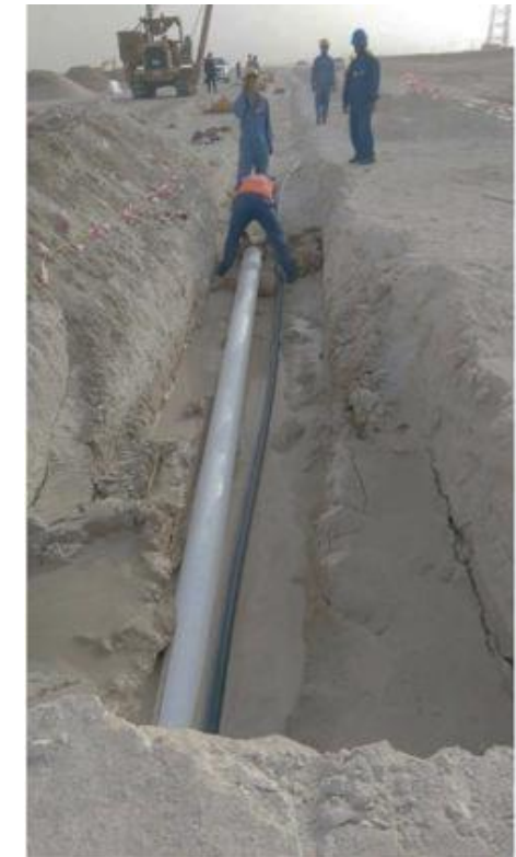
CO 2 pipeline with FOC
