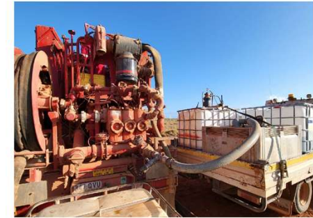
Rig-up from Chevron Barrow Island work, Australia
