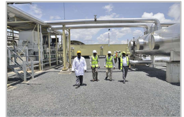
GEG and KenGen officials, 84 MW wellhead power plants, Olkaria, KENYA
