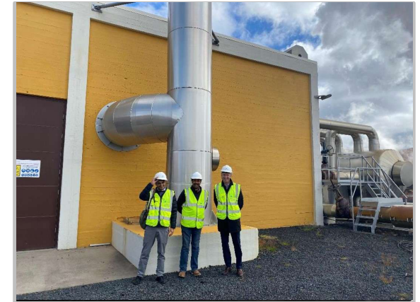
Bjarnarflag: 5 MW back pressure power plant, ICELAND
