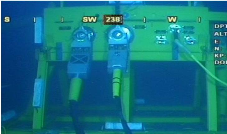
High-flow chemical delivery
